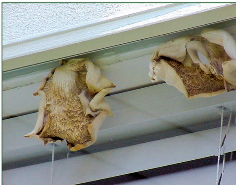
Photo 1: Previously undetected moisture is revealed through mushroom growth in a homeowner’s window.
