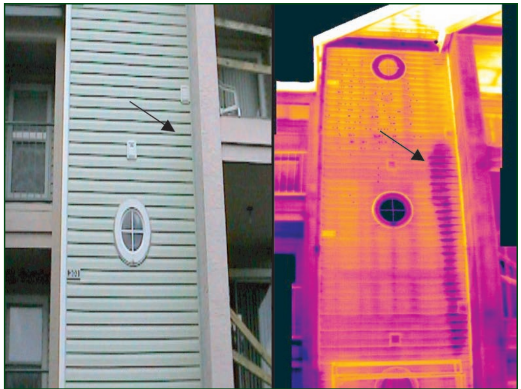
Photo 2 (left) shows apparently well-constructed exterior wall. Photo 3 (right), using an infrared camera, shows moisture infiltration not detected by the naked eye.
